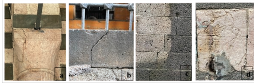
Figure 5. Capillary and Structural Crack Formation a. Corbel on the Arch on the North Façade b. Window on the West Façade c. West Façade Wall d. East Façade Wall
