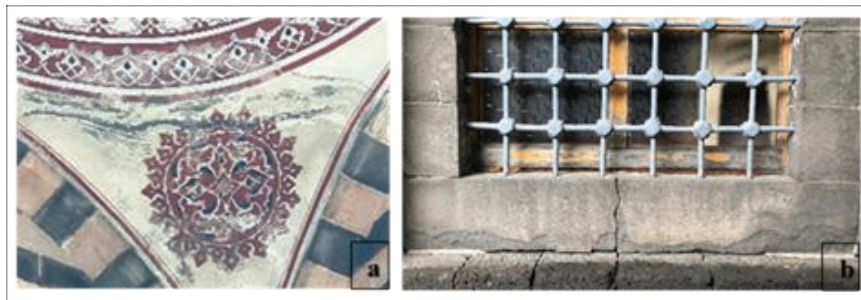
Figure 12. Scaling/Peeling a. Pendant on the North Façade b. Window on the South Façade
