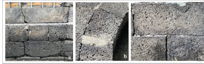
Figure 8. Mortar Erosion a. South Façade Wall b. South Façade Arch c. South Façade Wall
