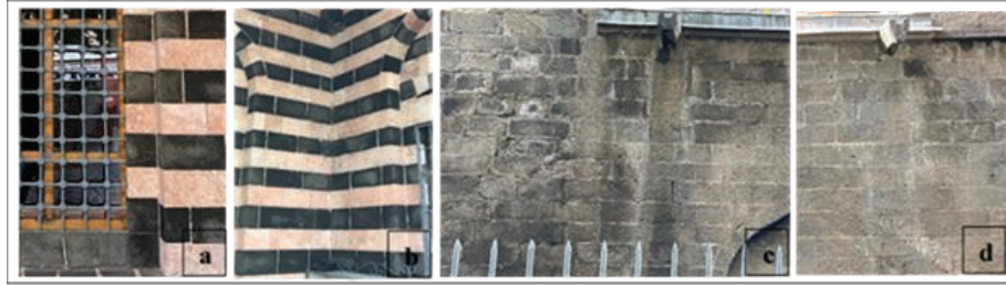
Figure 11. Efflorescence/Salt Crystallization a. North Façade Wall b. North-East Façade Wall c. West Façade Wall d. East Façade Wall
