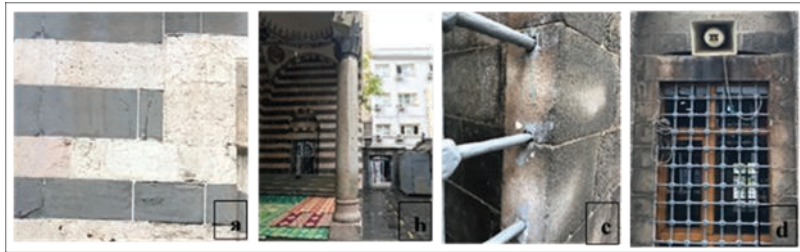
Figure 10. Black Crust a. North Façade Wall b. The column on the North Façade c. West Façade Wall d. Window Lintel on the West Façade
