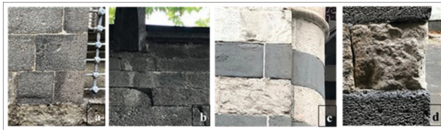
Figure 7. Abrasion / Loss of Surface a. Mausoleum Wall on the East Façade b. West Façade Wall c. North Façade Wall d. Minaret Wall on the West Façade
